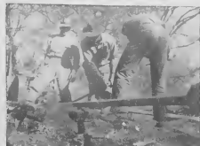
Portable suction lines are installed to save some of the oil that has leaked away. It will be pumped back into the main line. Other crewmen repair the damaged pipe.
